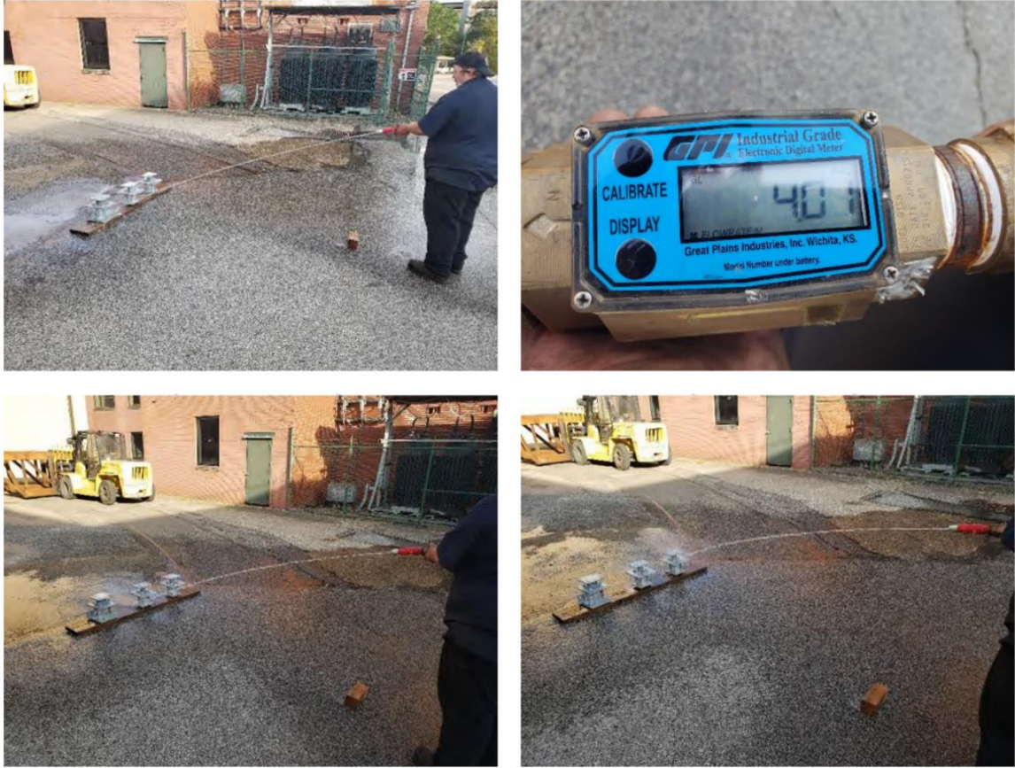
Figure 5: Water Ingress In-Process Testing
