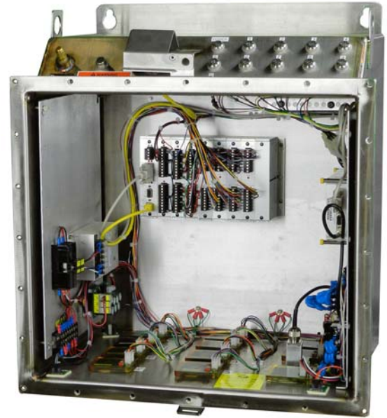
Current monitoring assembly with inputs from 30 CTs (10 circuits)
