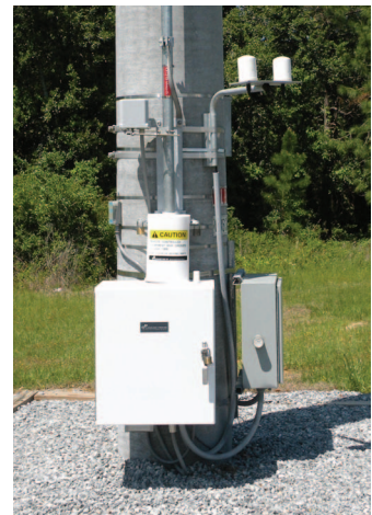
SCADA installation with BT-T motor operator and communication by radio.
