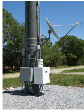
SCADA installation with BT-T motor operator and communication by satellite.
