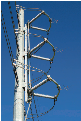
138 kV, 3000 A. "Quick Install" center break switch with porcelain insulators and quick break whips, mounted on a steel pole.
