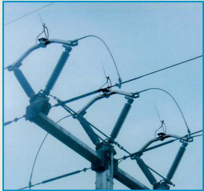
The Polywhip™ interrupter shown on a 138 kV CB-AV switch.
